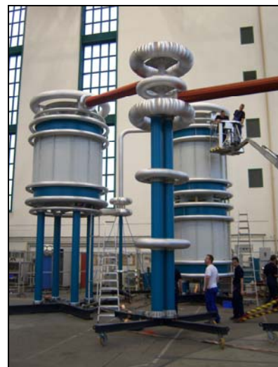
Fig. 5: Cascade of three tunable reactor modules
