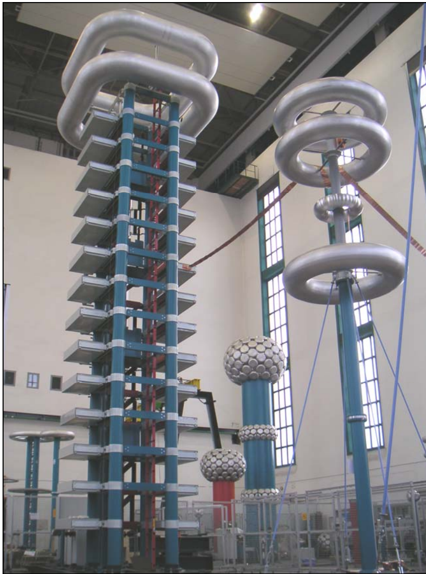
Fig. 2: Parallel overshoot compensation in front of impulse voltage generator
