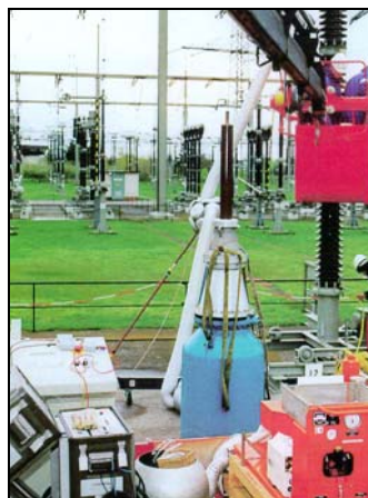
Fig. 4: SF 6 -insulated reactor with bushing to air
