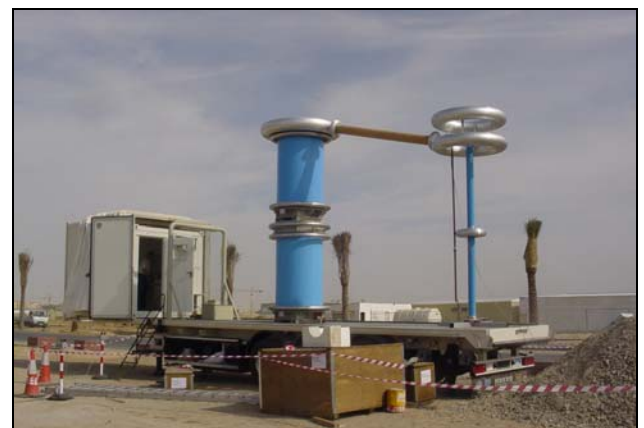
Fig. 5: Trailer with a modular test system: type WRV 3.8/600 M based on DEI reactors.
