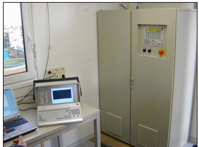
Fig. 1: Inside a control container for a frequency-tuned resonant test system for cable testing
