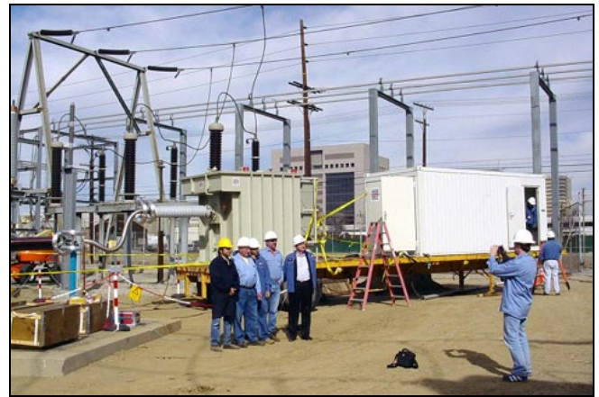
Fig. 3: Combined container on a trailer for HV cable testing (The exciter transformer is arranged inside that container).
