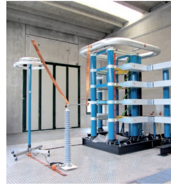
Fig. 3 Multi-stage Impulse Voltage Test System with modification to generate impulse currents
