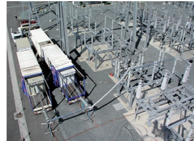
Fig. 3 On-site cable testing with HiRES Locator and AC resonant test system WRV 83/260 T
