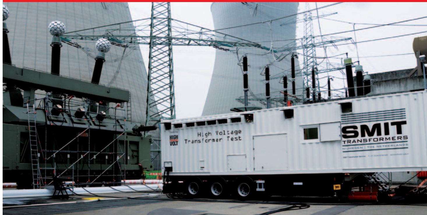
Fig. 1 On-site transformer test of a 1100 MVA unit at nuclear power plant
