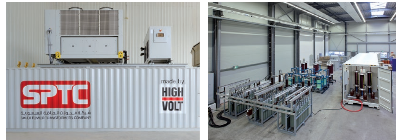
Fig. 3 Test system for medium power transformers (left: test voltage source 1 MW/2 MVA [SFC] in 40 ft container, right: test system 620kW/1MVA + HVCC)
