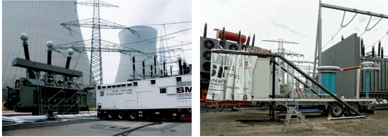
Fig. 4 Test system for on-site tests on transformers (left: WV 620-1000/80, right: extension for applied voltage tests WRV 5/360 M)
