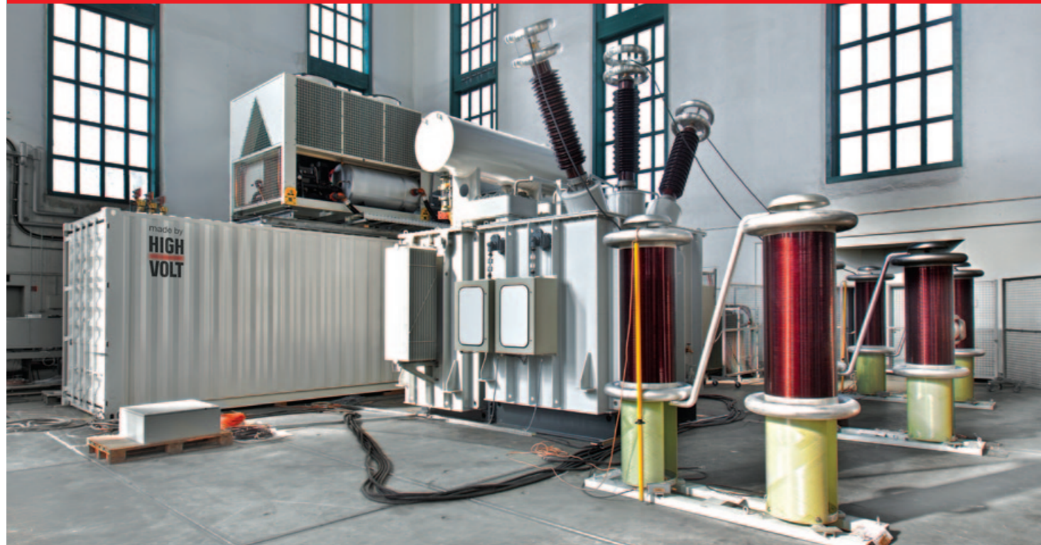
Fig. 1 Transformer test system for induced voltage tests, based on static frequency converter, type WV 2000-4000/170
