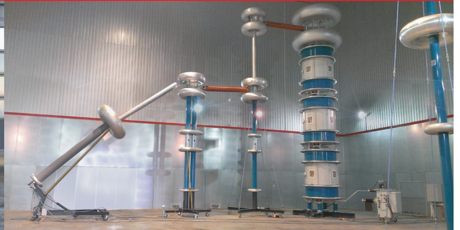
Fig. 2 Shielded room SSC 35x26x17 (incl. optional features) with integrated AC resonant test system WRM 5570/800 for type testing of high-voltage cables
