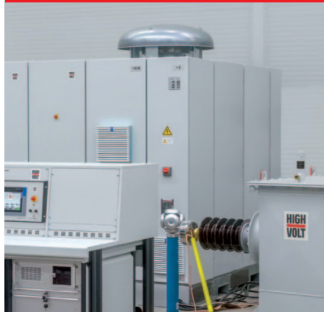
Fig. 1 Fully automated control system and frequency converter
