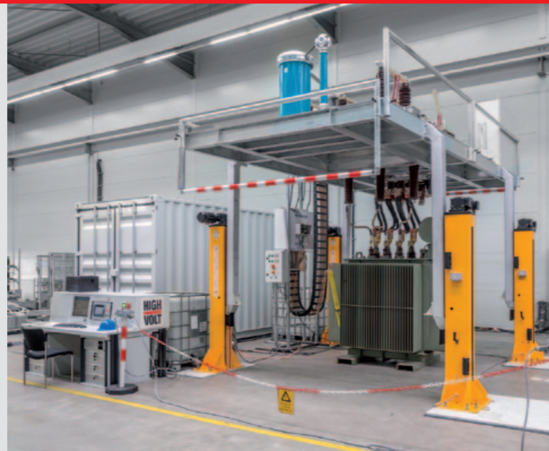
Fig. 2 Example showing the practical implementation of a customer-specific automatic switching system with height adjustment
